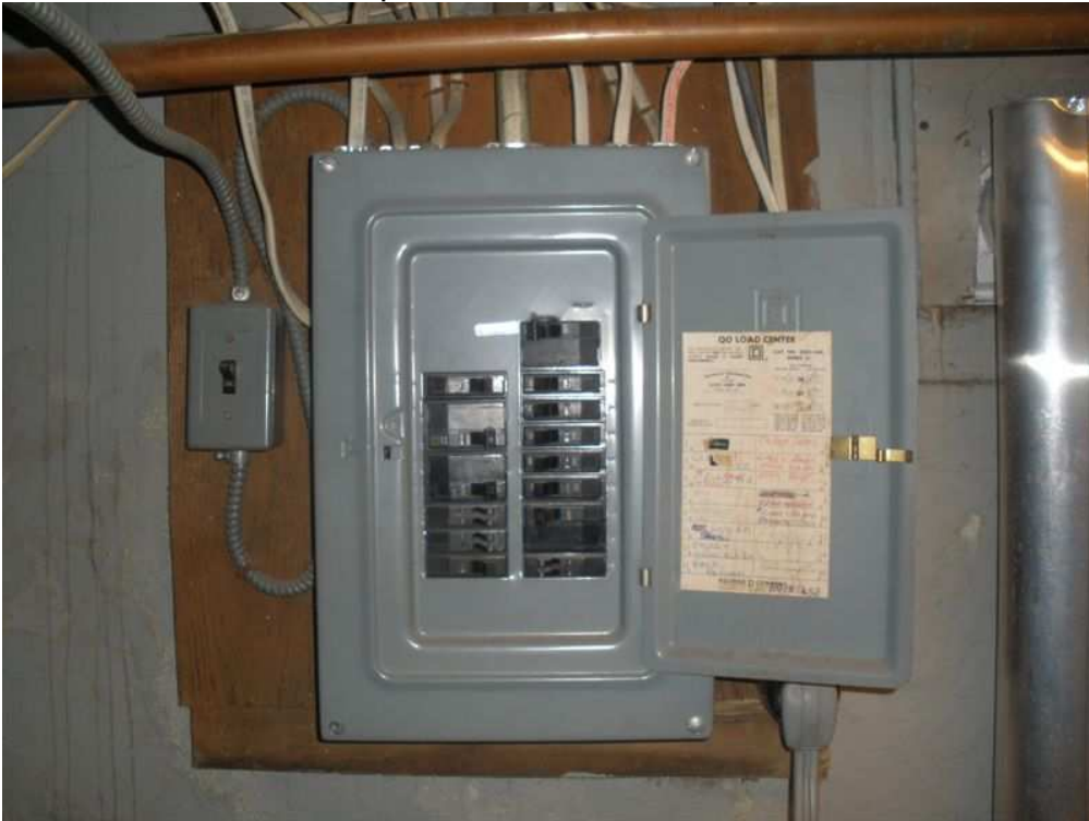
Photo # 17 main service panel
