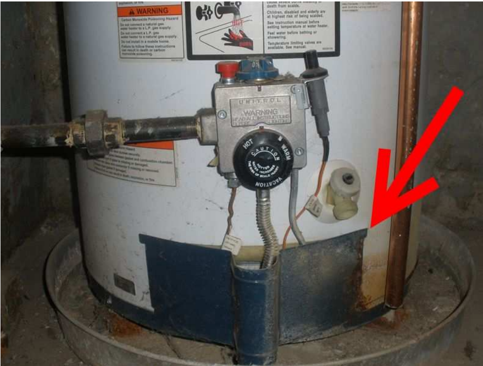
Photo # 14 water heater corrosion
