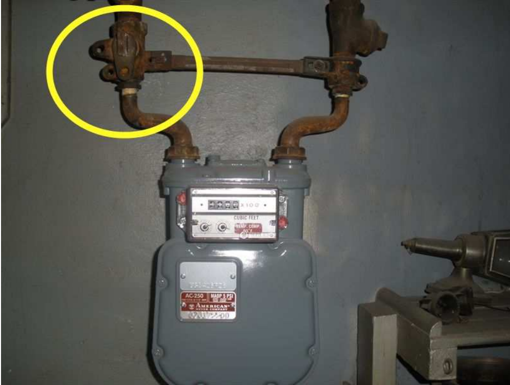
Photo #11 natural gas meter
