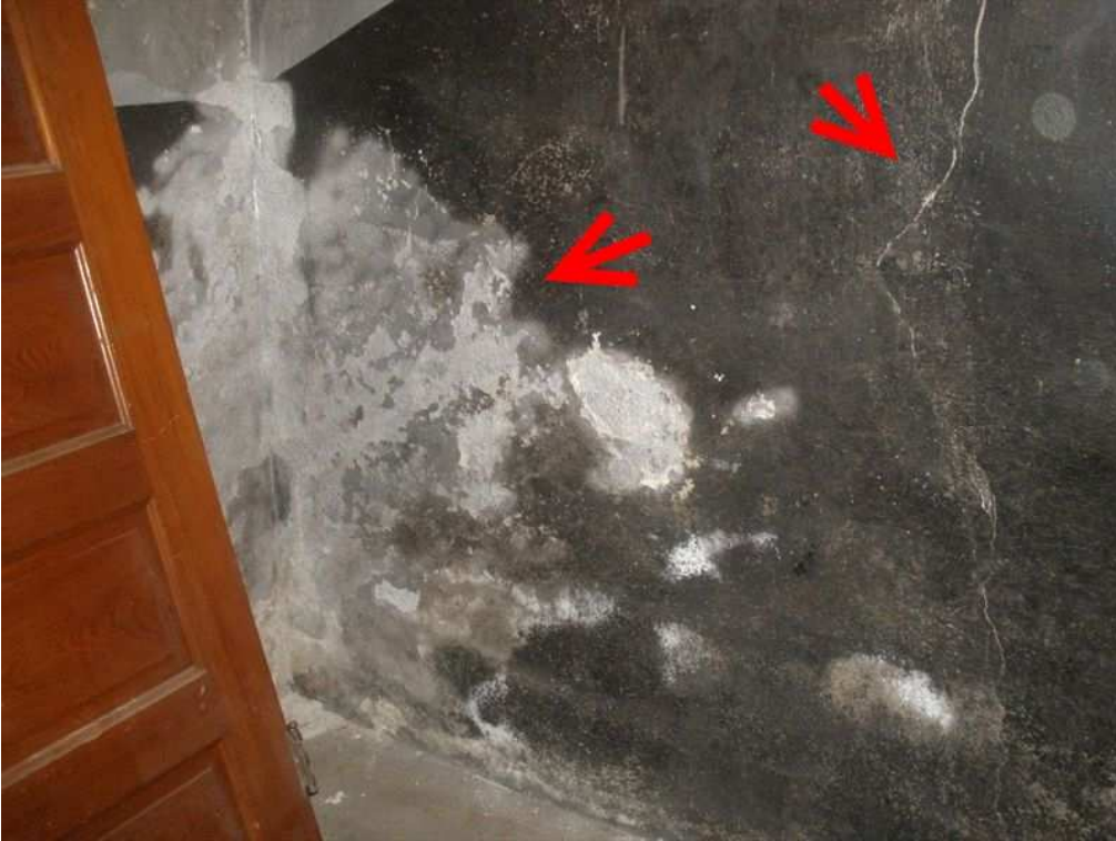
Photo #21 foundation water damage
