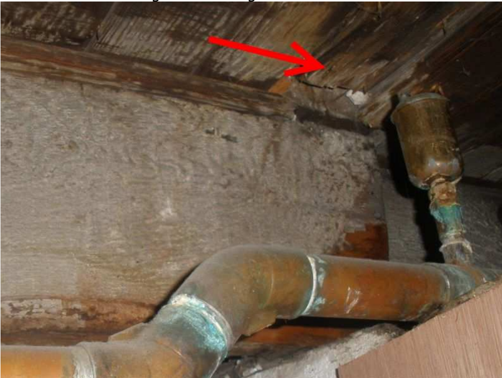
Photo #22 sub flooring water damage
