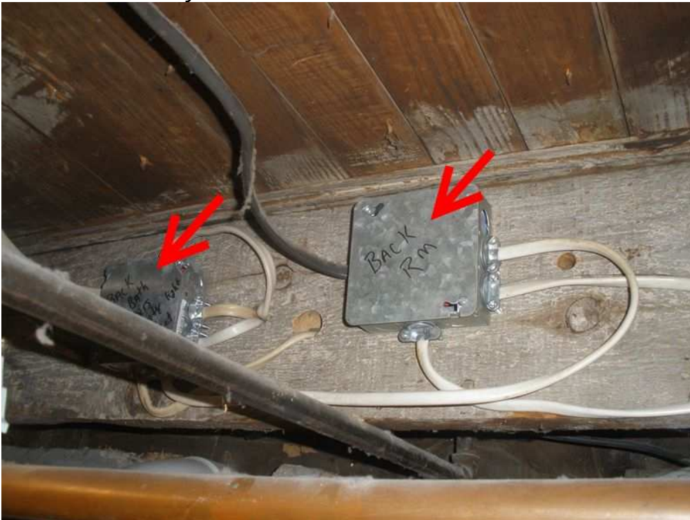
Photo #18 marked junction boxes
